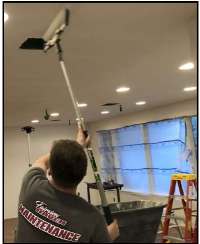
REMODELING of the living room and front entrance is almost finished, thanks to the hard work and dedication of our maintenance crew and contractors. Here's Jeremiah Rinkenberger painting the living room ceiling on a Saturday night.
